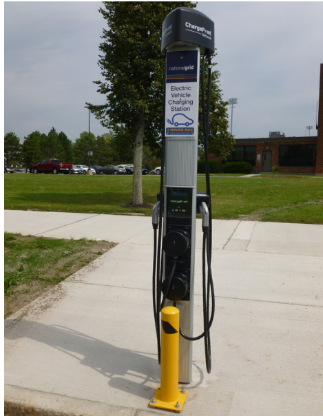
Level 2 charging station at Bissell Hall on University of Buffalo's North Campus. Photo credit: Energetics
